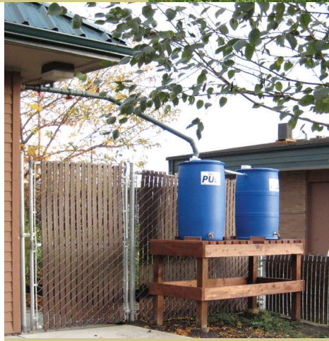
Rain barrels capture roof rainwater for irrigation at the Skagit County Administration Building
